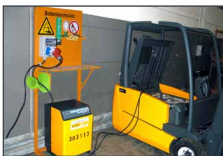
Station de charge de batteries
